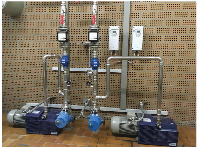
Fig. 4: The DG1 drives are also used to aerate the well water.
