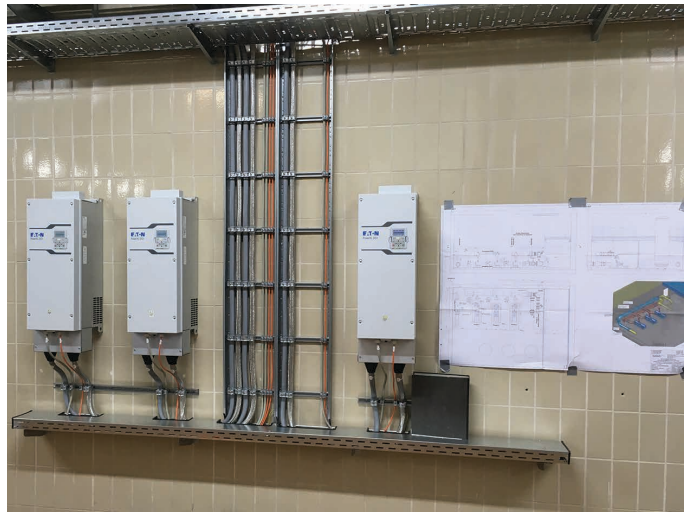
Fig. 3: The application is now speed-controlled, thanks to the combination of IE4 motors and DG1 drives. The power losses associated with the old gate-valve system have thus been eliminated.
